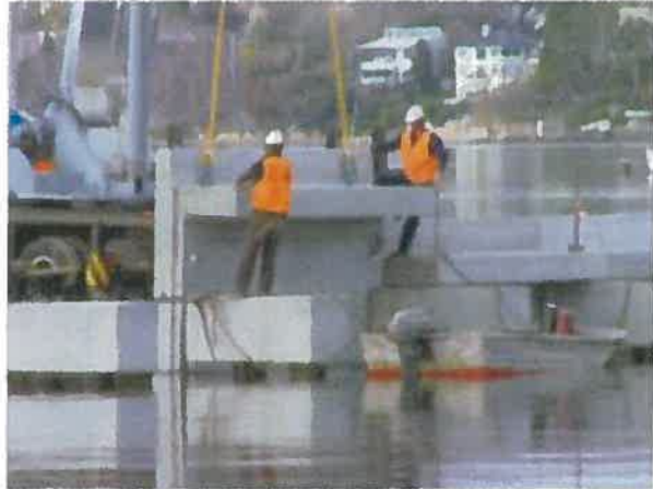
Photo B: Construction of fixed panel wave attenuator – showing fixed panel being positioned onto pile caps
