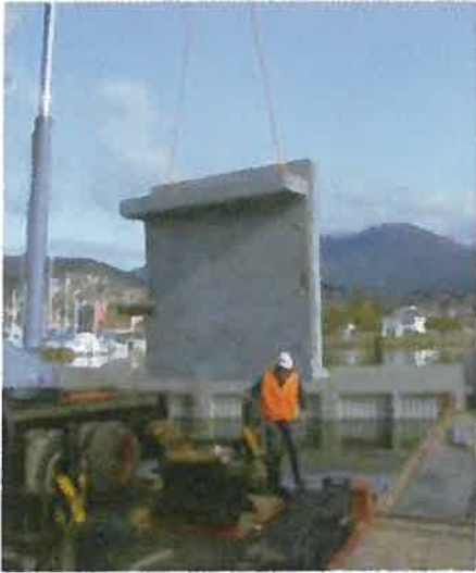
Photo A: Construction of fixed panel wave attenuator – showing fixed panel being lifted into place by floating crane.
